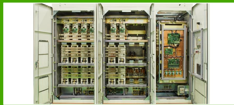
Accelerator power supplies
